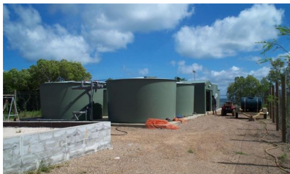
Saibai Island sewage treatment plant.
